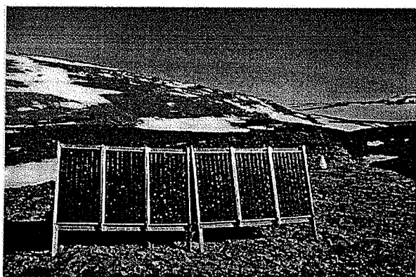
Fig. 5. Setup of the equipment at Beaver Lake in 1999. The GPS receiver and batteries are in a plastic suitcase behind the solar panels, while the GPS antenna and radome can be seen on the ground behind and to the right of the panels.
